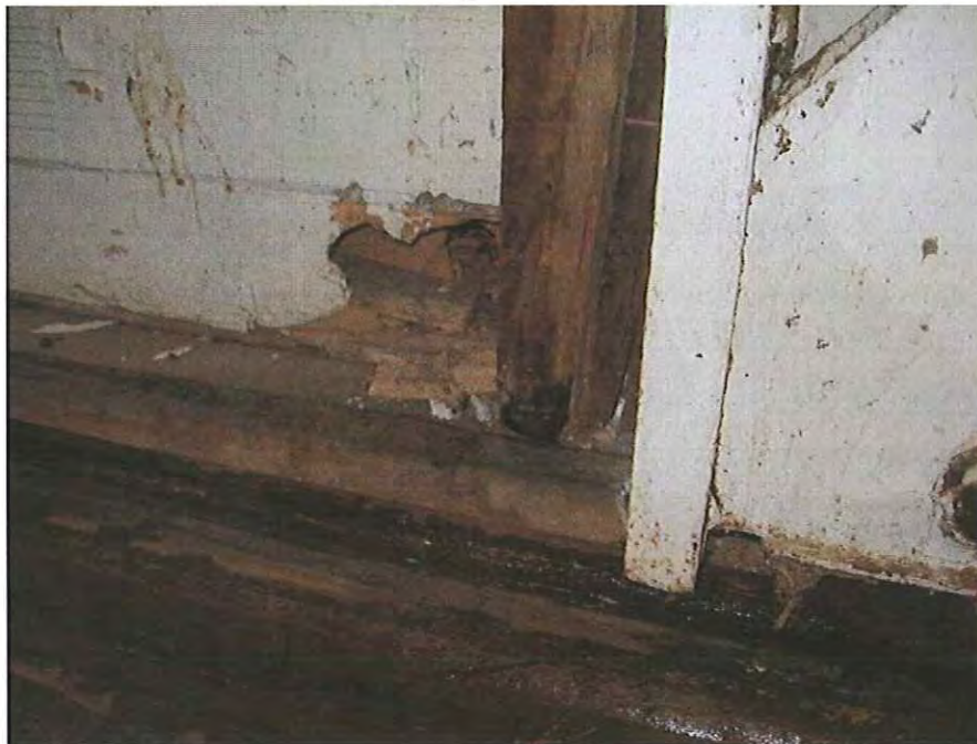
16. Bottom of wall on west side of hangar door is damaged.
