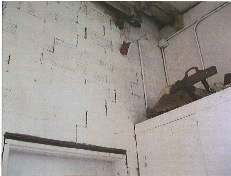
18. Step cracks at top of wall on east side of hangar door.
