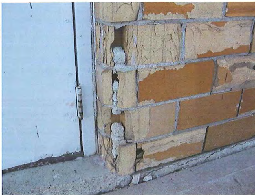
5. Clay tile is in poor condition near the northwest walk door.
