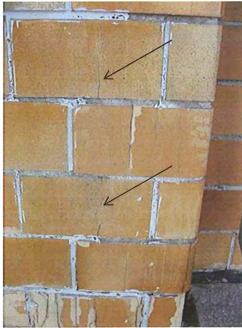
7. Cracks are present in clay tile.
