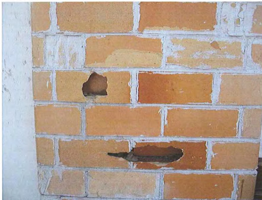
8. Holes are present in exterior wythe of clay tile.
