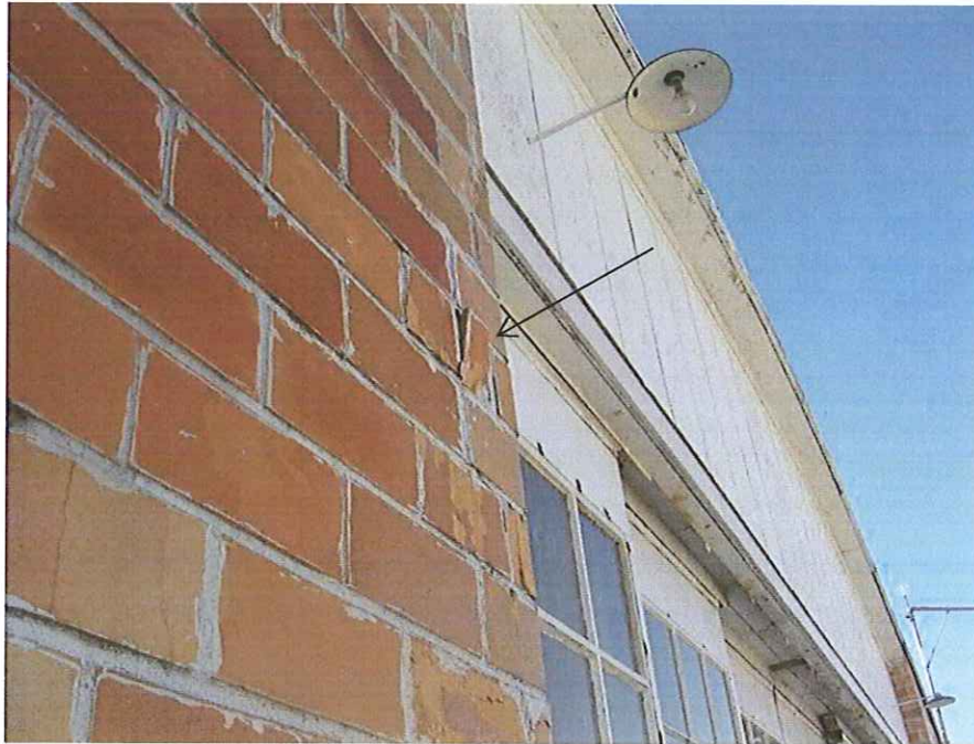
9. Portions of clay brick are falling off building.
