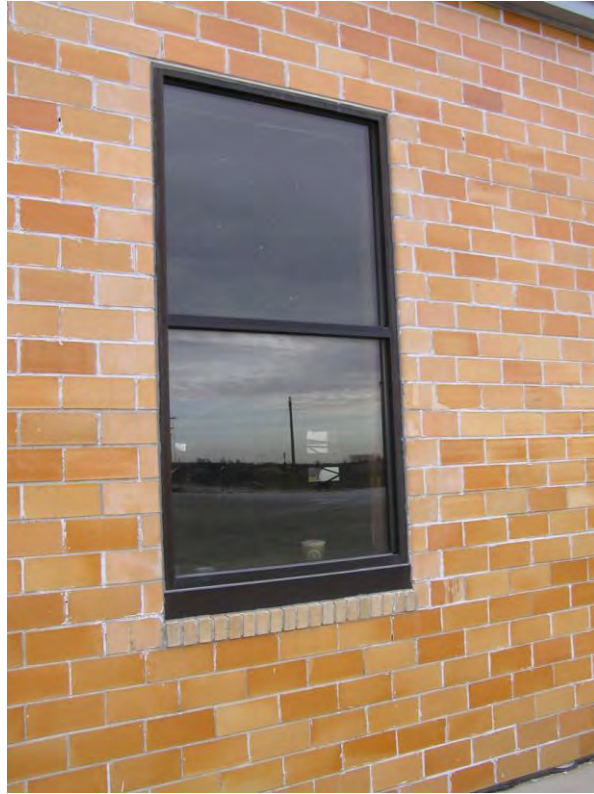
PHOTOGRAPH 4. View of Metal 2/2 fixed replacement windows on Building A. Note the modification to the window opening.
