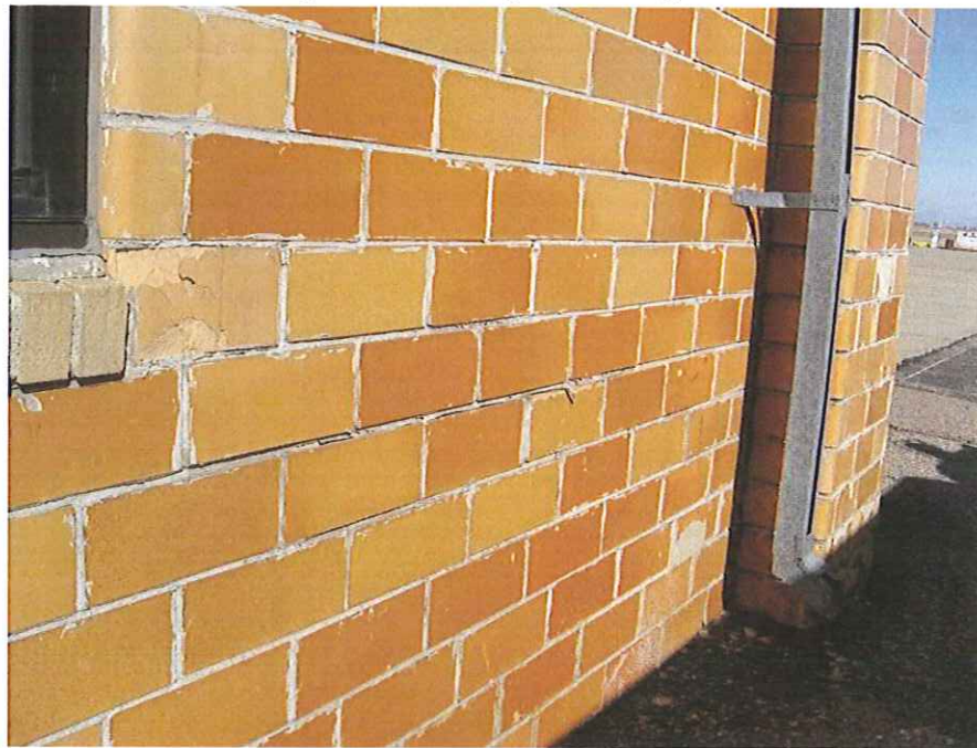
10. Tuck pointing that has been done has deteriorated.
