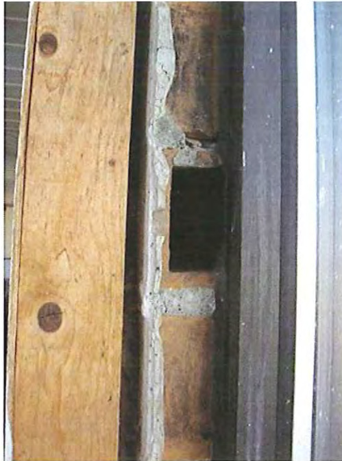
15. Interior stud wall, sheathing and cross section of clay brick at window.
